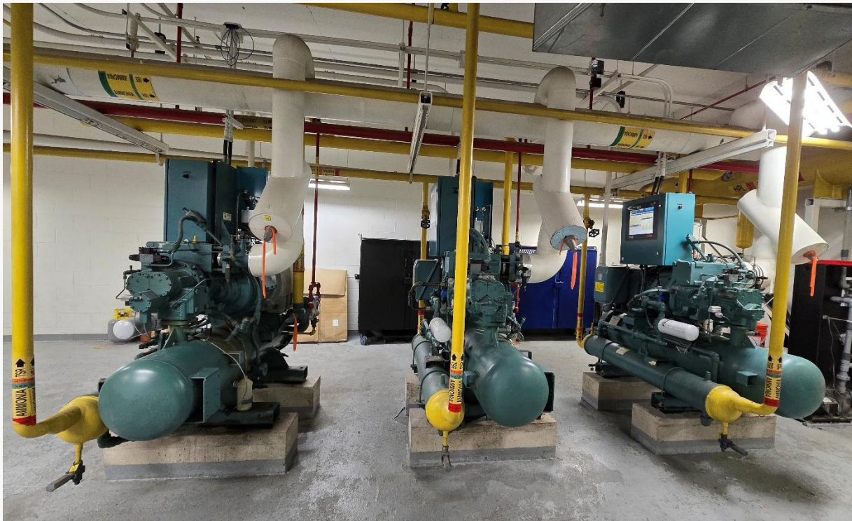
FIGURE 4.5: Three screw compressors in refrigeration unit
