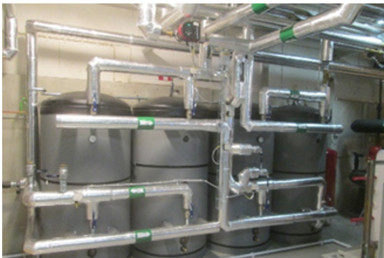
Figure 38. Groups of accumulator tanks with coils for tap water pre- and post- heating.
