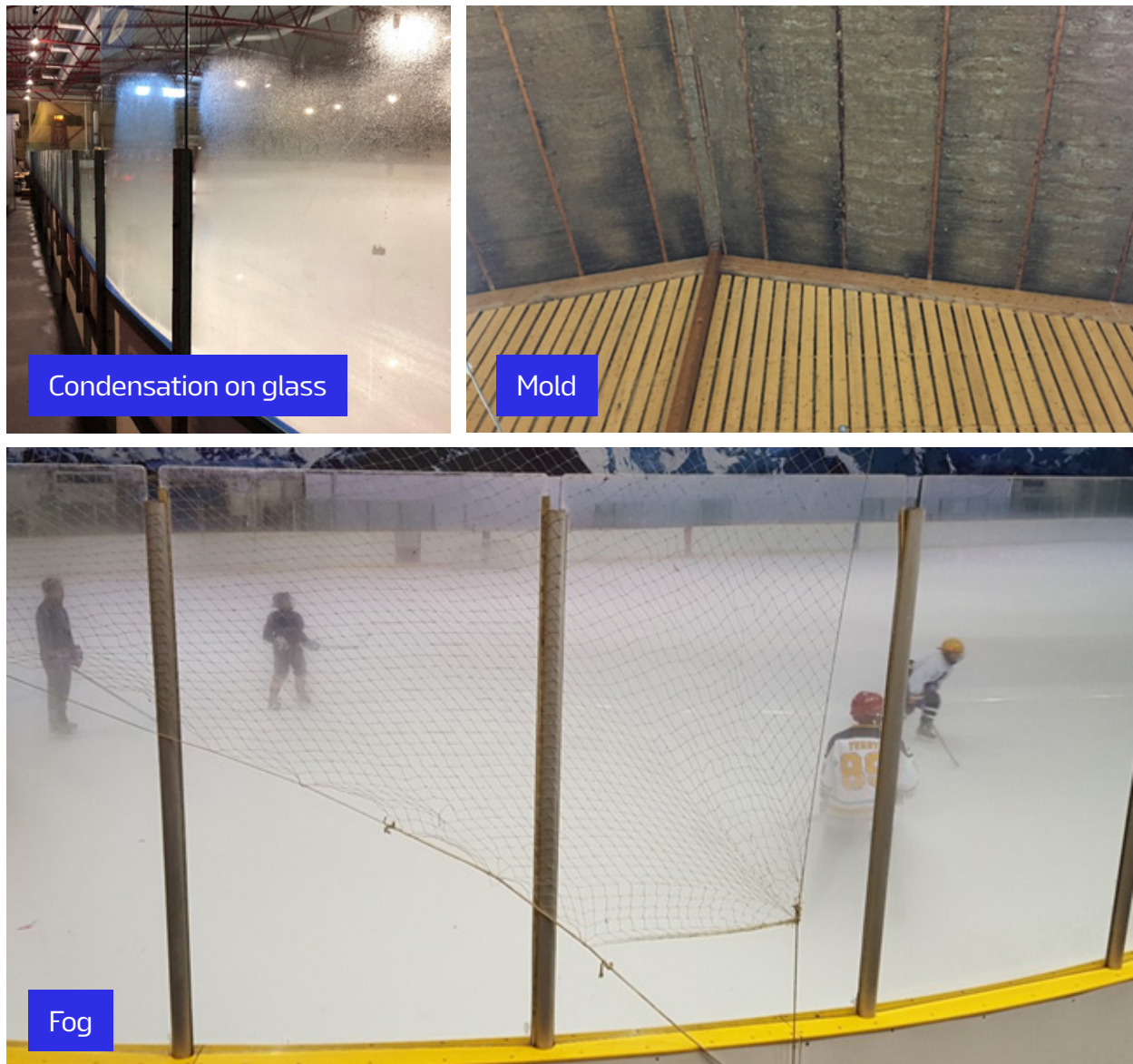
Figure 40. Moisture problems are known in many ice rinks. Solution to keep the indoor humidity at acceptable level must be used.
