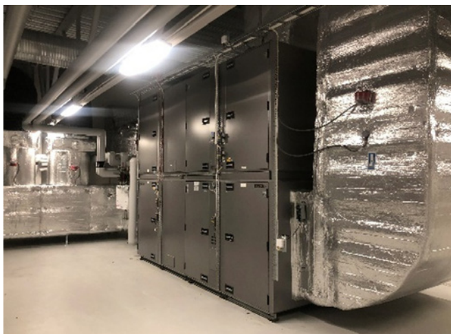
Figure 52. Example of a central air handling unit in an ice arena, the unit is located in a technical room.
