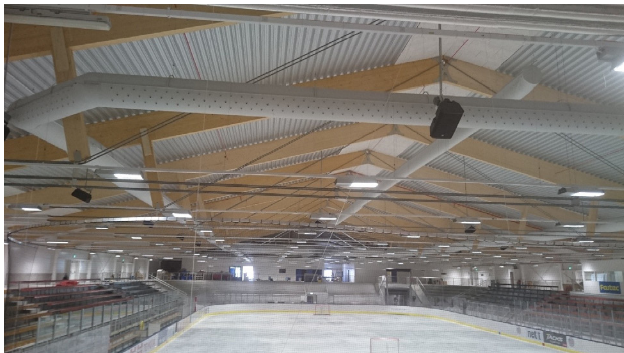
Figure 50. Textile ducts in an ice rink where dry air is distributed over the ice and “comfort air” to the stands.
