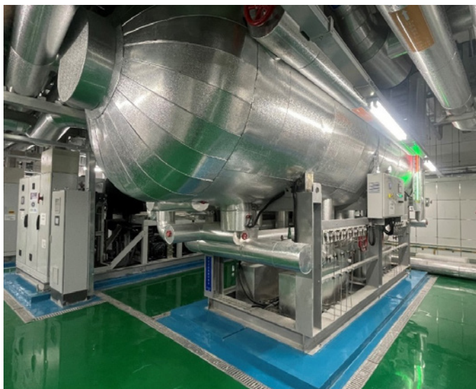
Figure 32. CO 2 receiver in a large ice arena where CO 2 is circulated in the rink piping [NSSO, Beijing].
